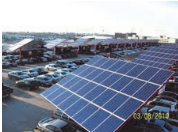
Figure 2.7: Pole-mounted PV system at Logan Airport.
