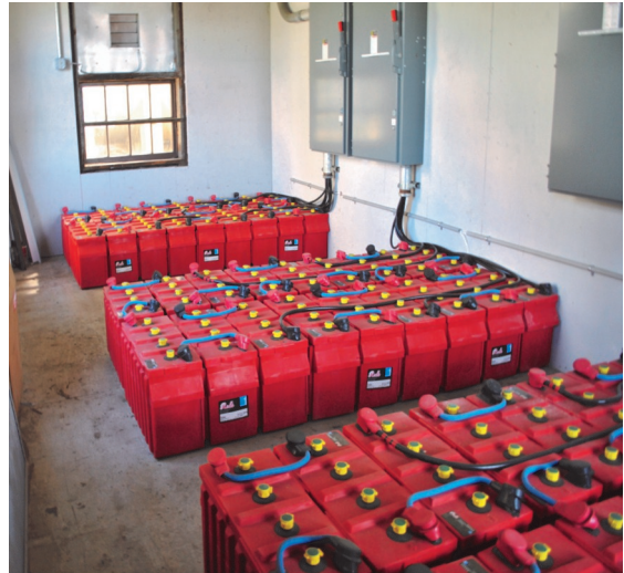
Fig. 2.3. A battery bank for an off-grid PV system on Georges Island in the Boston Harbor Islands.
