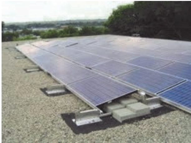
Figure 2.6 Commercial ballasted PV system on the Roosevelt Elementary School.
